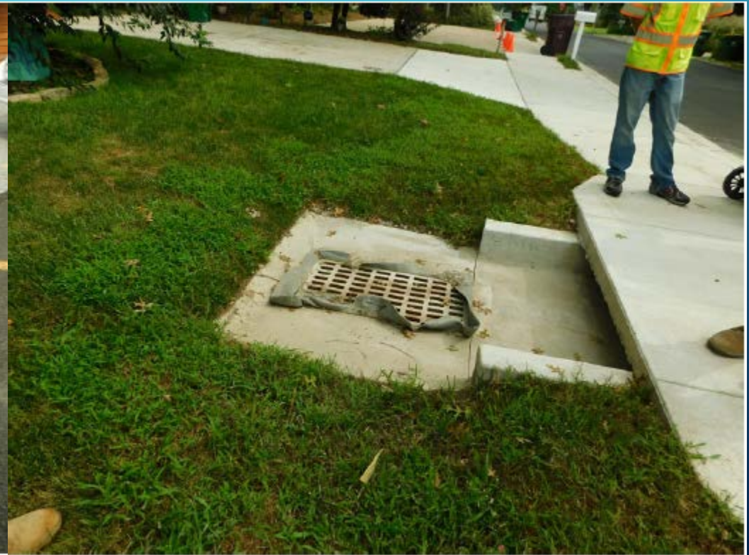
Poor use of Type 3 Grate
